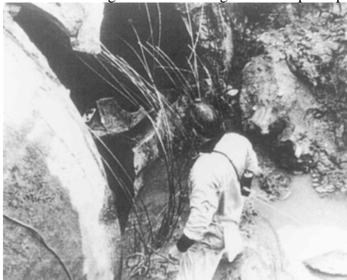
Fig. 8 Damage due to prestressed concrete cylinder pipe burst (Mojave Desert)
