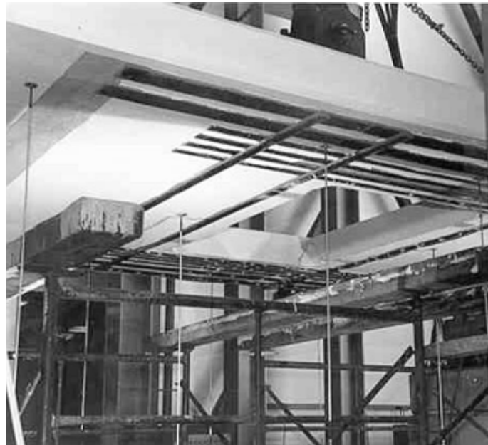
Fig. 7 Placement of composites around cutout in slab to provide external reinforcement for stress redistribution
