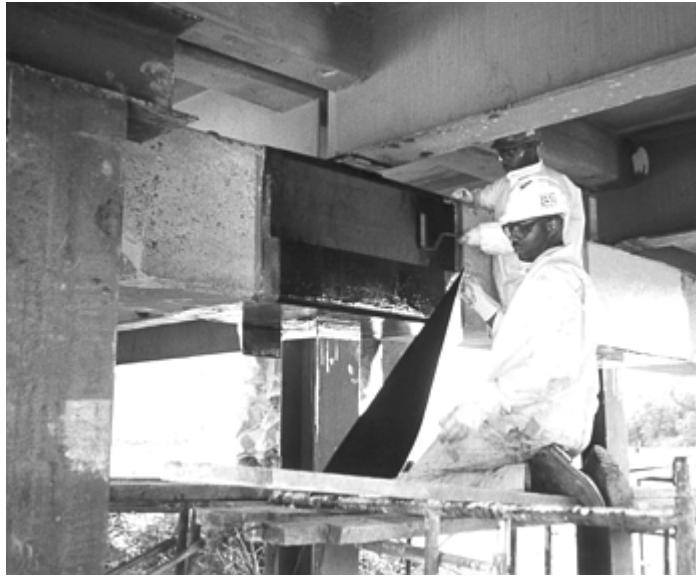
Fig. 13 Fiber-reinforced polymer sheet applied to the side of a beam to increase the shear strength of the beam
