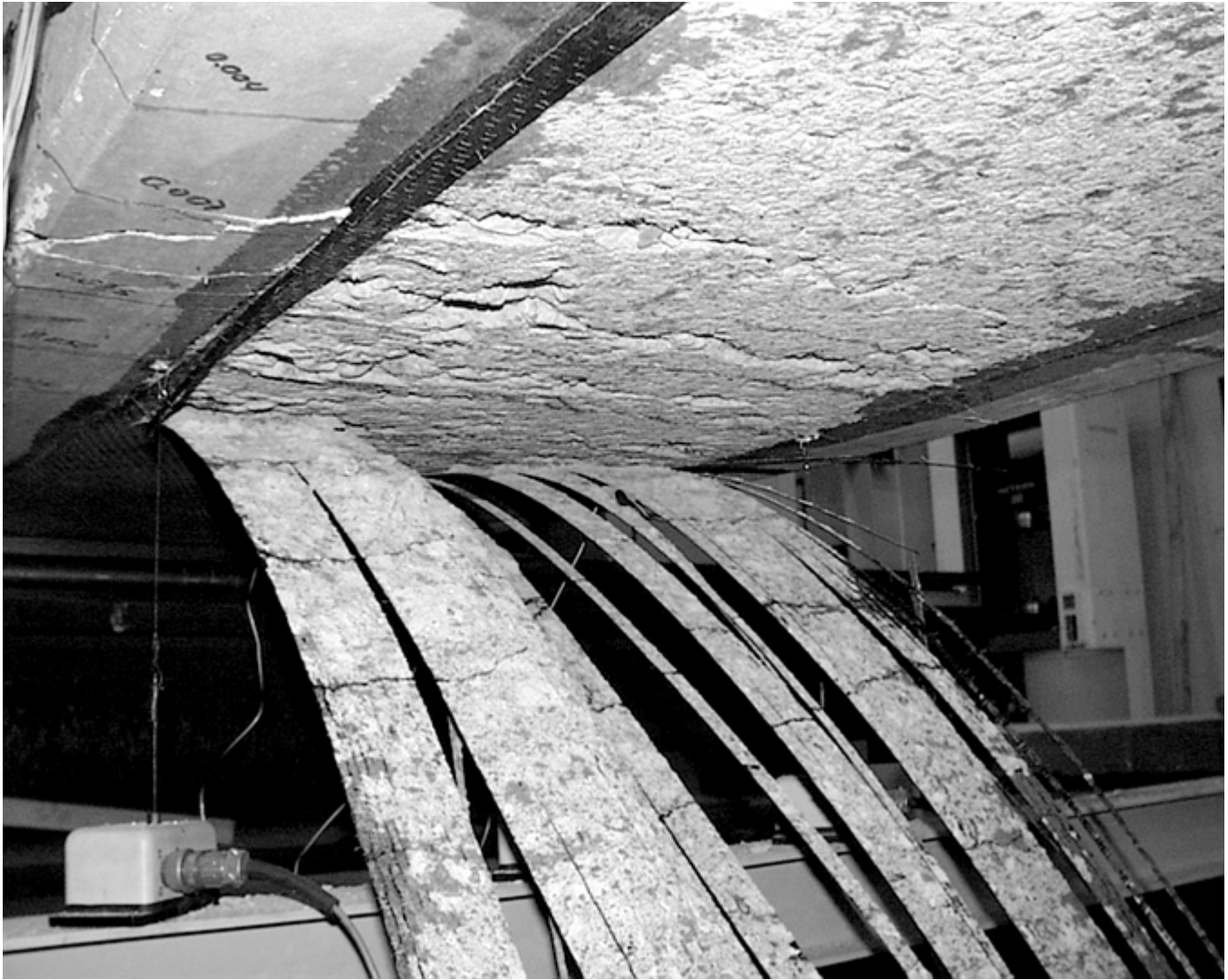
Fig. 12 Delamination of fiber-reinforced polymer composite from concrete slab in flexural failure. The concrete remaining on the composite indicates good bond.
