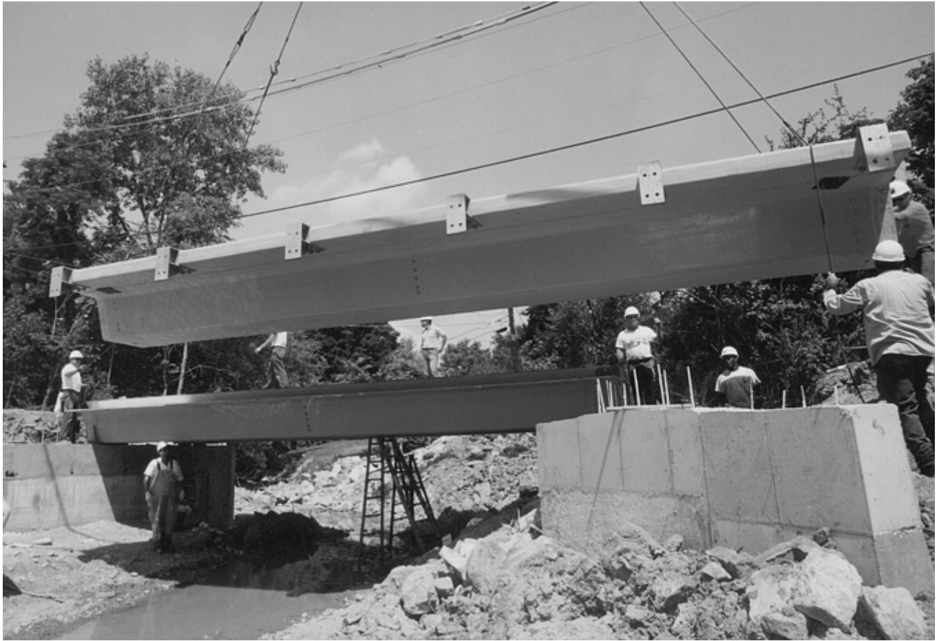
Fig. 4 All-composite bridge in Butler County, Ohio. Factory-constructed primarily using glass fiber, the bridge was trucked to the site and installed in less than one day.
